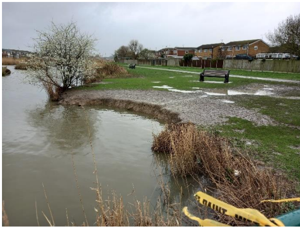
Bank erosion on the southern side of the lake
